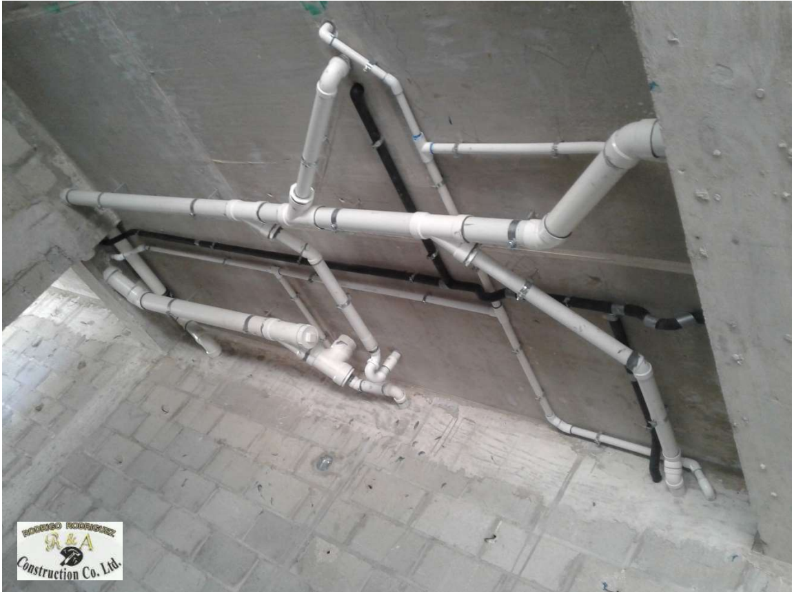
FIRST FLOOR PLUMBING ON GROUND FLOOR CEILING - FINCA SOLANA
