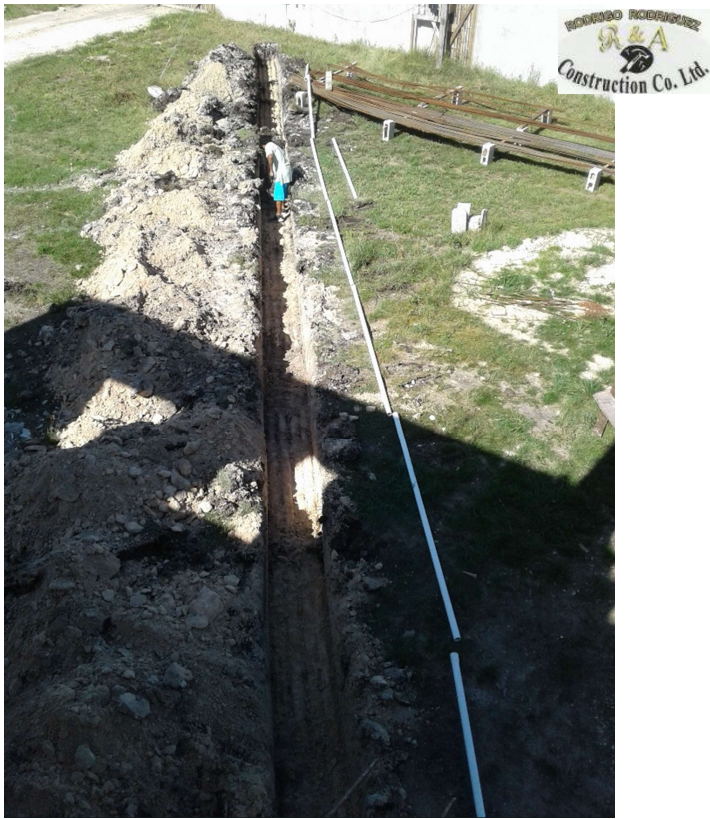
ELECTRICAL MAIN LINE TO BUILDING - FINCA SOLANA
